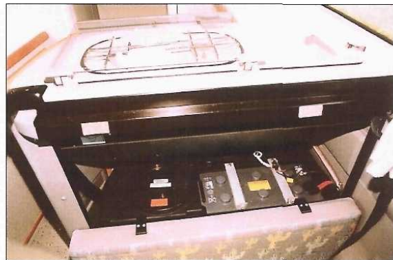
Under the kitchen (with cushion removed) you can see the gas locker (left) and auxiliary battery (right). Waste water tank is also here.
